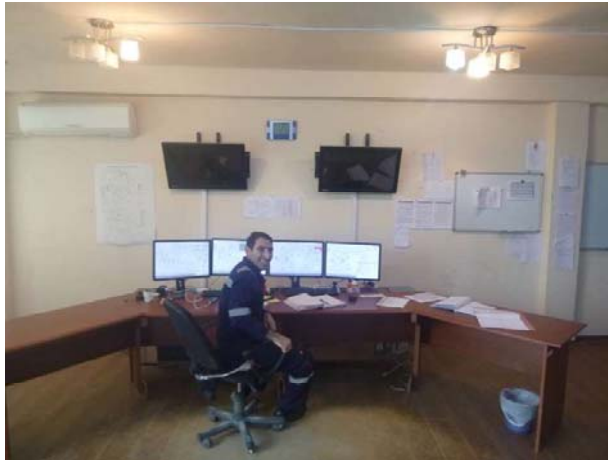
Figure 6 – Central control room for concentrator and Albion Process™ plant.
