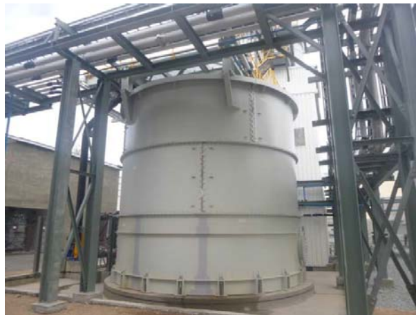
Figure 5 – Limestone storage tank.
