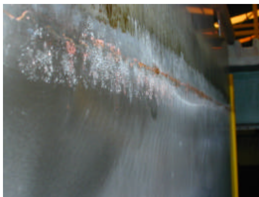
Figure 4: Solution line corrosion
